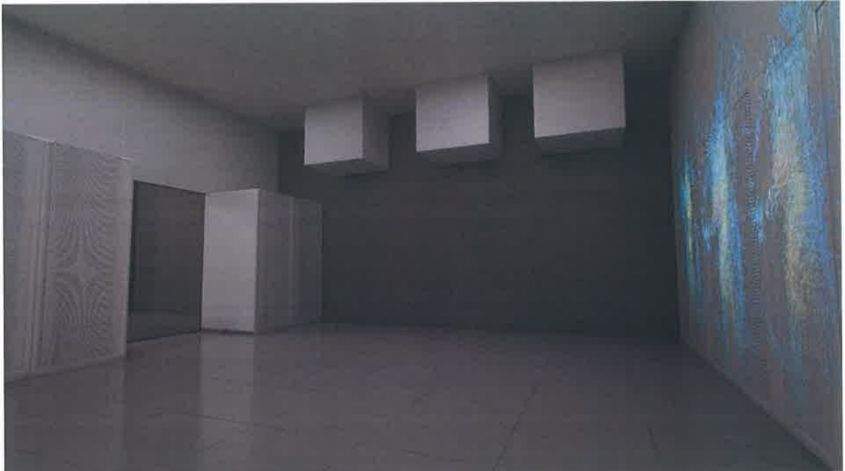
Cold zone with first row racks and AC units
